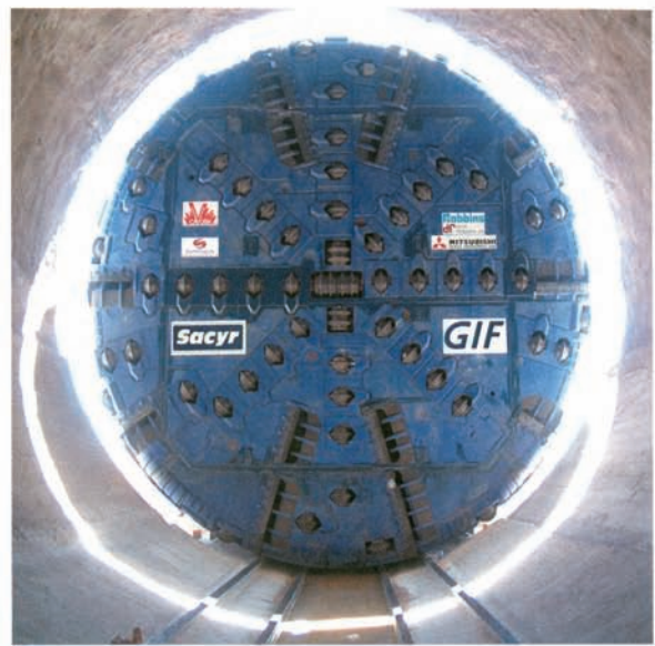
Foto 4 bis. Cabeza de corte de la TBM del túnel Oeste/Photo 4 bis. Cutting head of the TBM for the West tunnel before being assembled on site.
